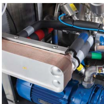
Multi-colour coded piping with isolation
